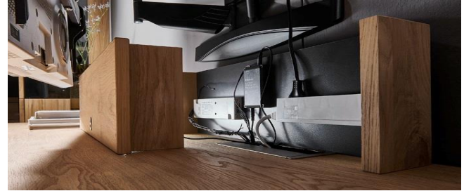
Fig. 2: Example of wiring
